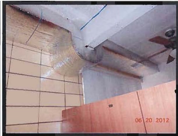
Close-up of HVAC Ductwork
