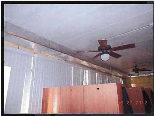
Overview of HVAC Ductwork
