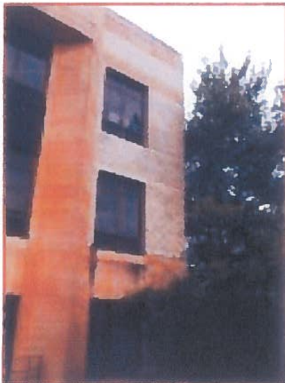
Sandstone Stain under Second Floor Window
