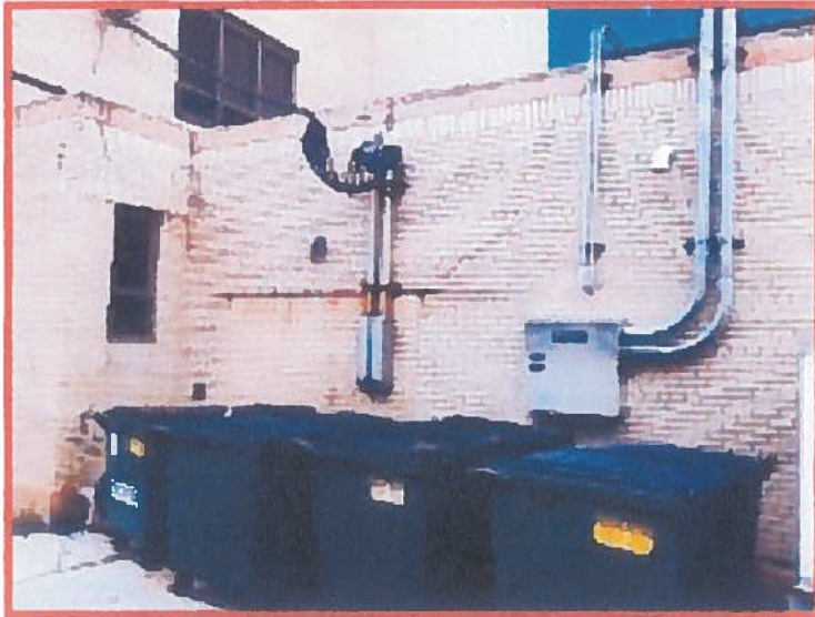
The Patched Door Area which Requires Repair.
