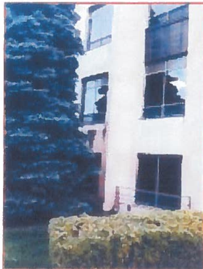
Sandstone Stain under Second Floor Window
